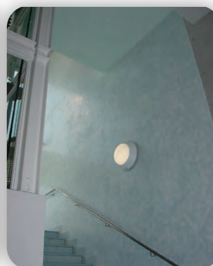
Polished Shikkui walls in a railway station
